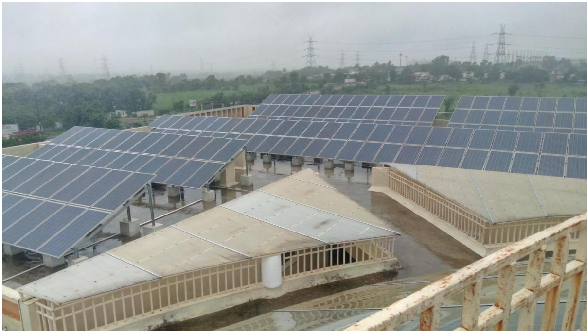
Rooftop Solar Photovoltaic Power Plant at CDGI
